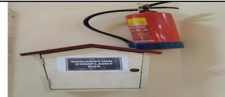
fire extinguisher , Suggestion and complaint box
