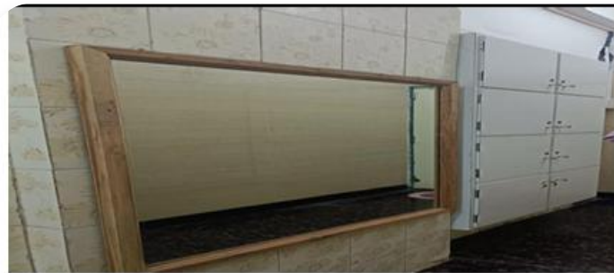
Mirror and locker facility in second floor ladies toilet.
